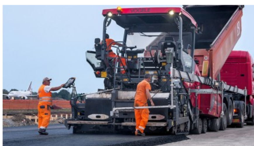
Ultra-modern, user-friendly technology is the basis for the innovative, environmentally friendly and economical asphalt pavers of the new "Dash 3" generation from Vögele. That also applies to the SUPER 1803-3 wheeled paver used in Bologna.
