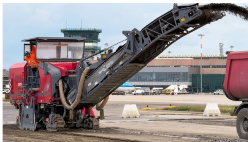
Located some 200 km southeast of Milan, Guglielmo Marconi Airport is undergoing extensive rehabilitation work. The paving courses were milled off by the Wirtgen W 200. Easy to handle, the lightweight large milling machine is among the all-rounders in road rehabilitation and boasts an impressive performance and cost-efficiency
